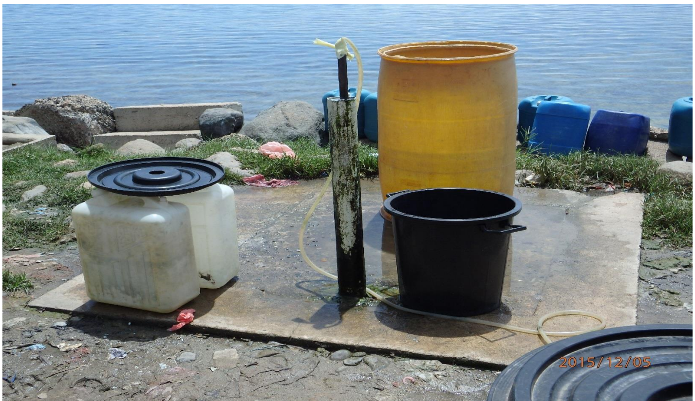
A stand pipe in the Malakerava area identified under the quick fixes for Gizo. This is an example of stand pipes requiring urgent attention to prevent water running 24 hours, 7 days a week. This is a popular water source used by business houses in Gizo. Business employees and local residences queue for hours to get water from this stand pipe during peak hours (some till early morning hours). Photo: Joy Papao, GIS Specialist, SIWSAP.
